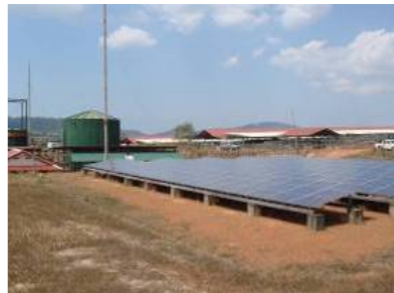
Figure 3: Local/Village grid fed by Hybrid 50 KWp PV and 35 kWe Biogas system, Cambodia
